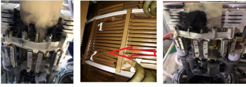
Figure 1. The basic situation of No.2, No.3 transformer
