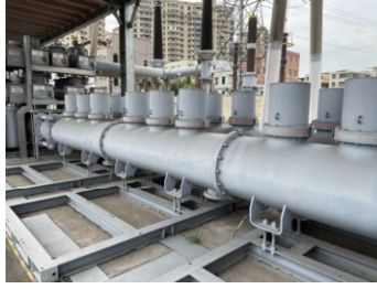
Fig.1 GIS Equipment Distribution
