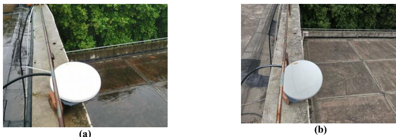
Figure 13. (a) The omnidirectional receiving antenna when it rains; (b) The omnidirectional receiving antenna when it not.
