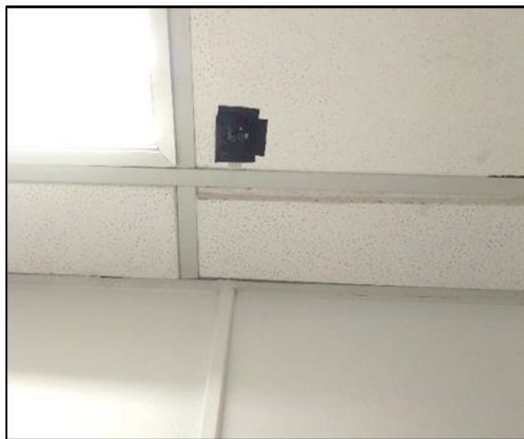
Figure 3. Camera installation in top view.
