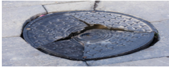
Figure 1. A damaged manhole cover
