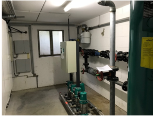
Figure 4. The Heating Room.
