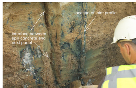
Figure 8. Typical double joint caused by spill concrete
