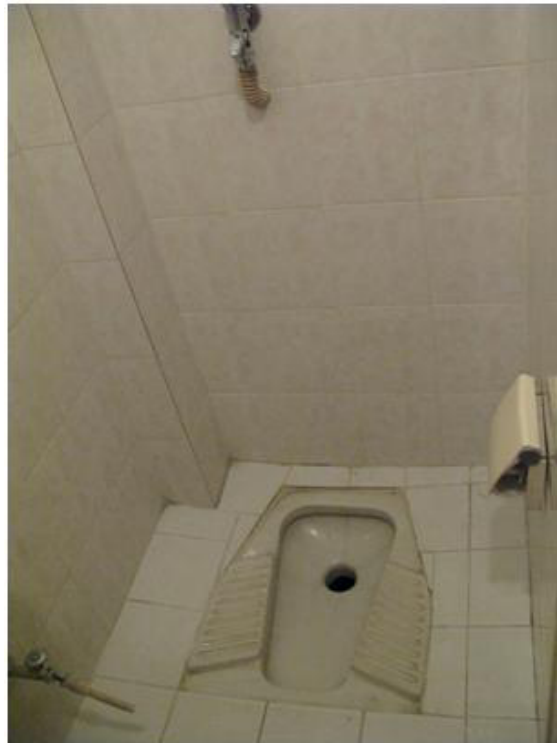
Figure 1. A typical Turkish squat toilet with a water tap on the right, a toilet paper roll holder and a wall mounted flush button.
