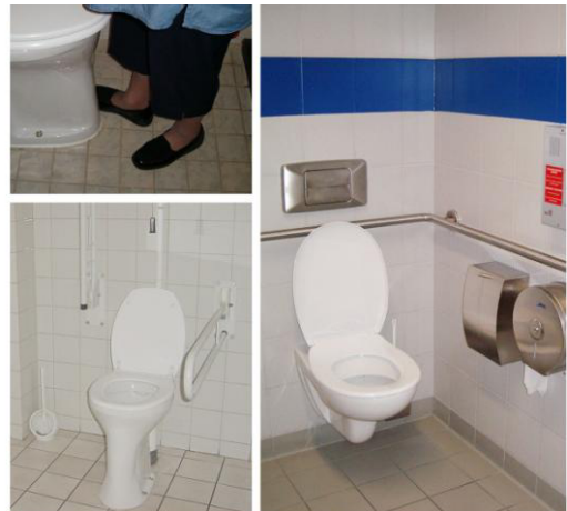
Figure 2. The toilet bowl as object to trip over (upper left), lack of contrast (lower left), visual support and a deceptively continuing floor (both on right)
