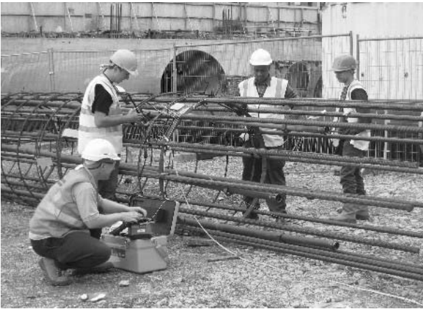
Figure 105. Installation of the BOTDR Fibre Optic sensor to the pile reinforcing cage at the Bankside Development.
