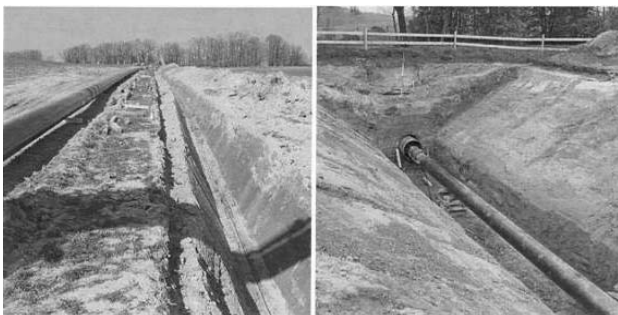
Figure 102. Construction of the brine pipeline, with FO sensor placed at 6 o'clock position (Nikles et al., 2004).
