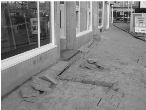
Figure 17 – Settlement caused by wash-out of deep sand layer.
