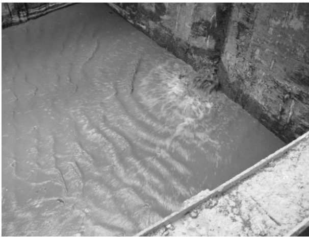
Figure 13 – Water and sand entering the excavation
