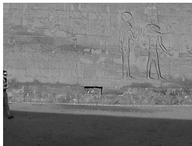
Figure 4. Deterioration of the temple due to groundwater rise
